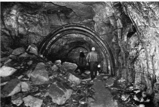
Roof falls, hooped railway lines showing how the tunnel would be finished, and all but blocked at the end. Thorsten Hintze examines the rubble while Sascha Keil advances.
